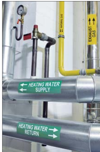
Large and highly visible pipe marking.
