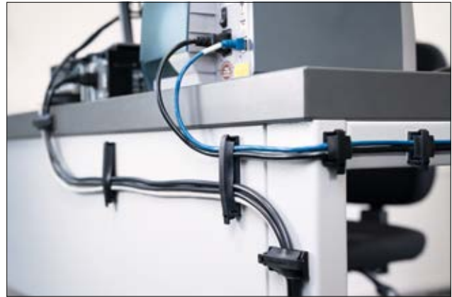
Perfect solution to route cables along the office desk.
