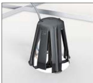
2. Push the spikes into the plasterboard to prevent shifting and disconnect the tool.
