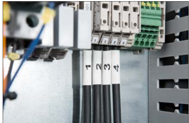
TLFD DS shrinkable markers for more safety and clarity in the switchboard.
